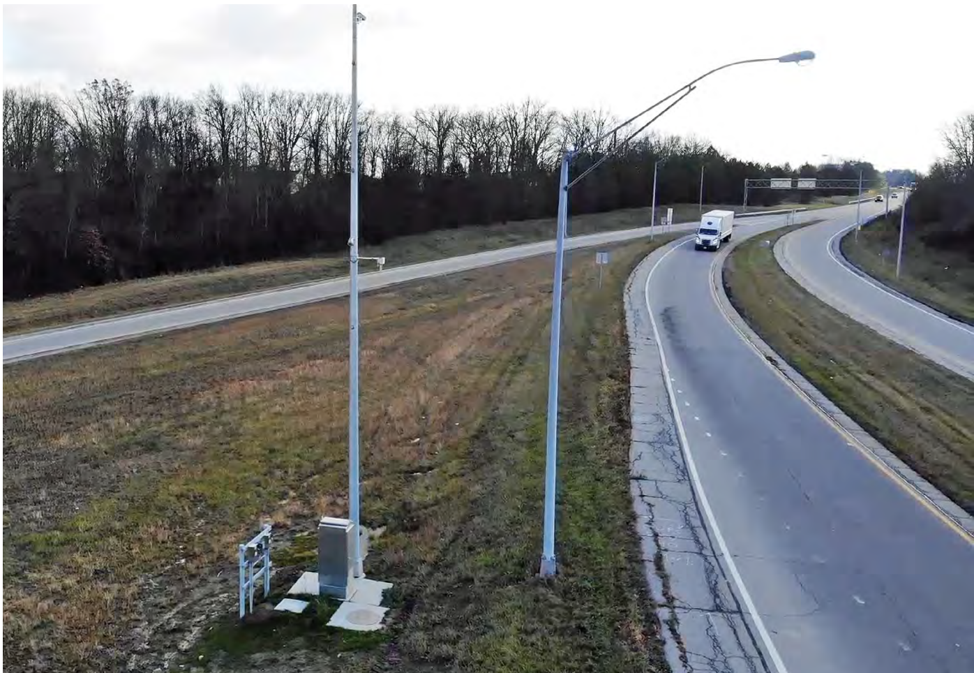
FIGURE 14: An RSU pole with ground mounted ITS cabinet.
