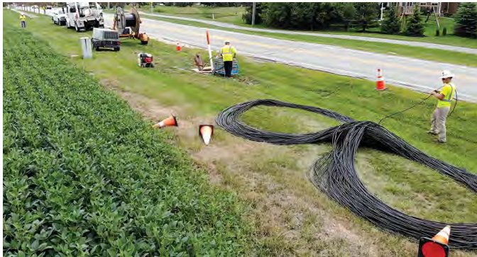
FIGURE 10: Shown are several thousand feet of micro cable ready to be air-jetted through the 7-way duct.
