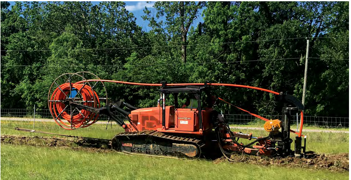
FIGURE 9: In addition to directional drilling, vibrate plowing methods were used to install the 7-way duct.
