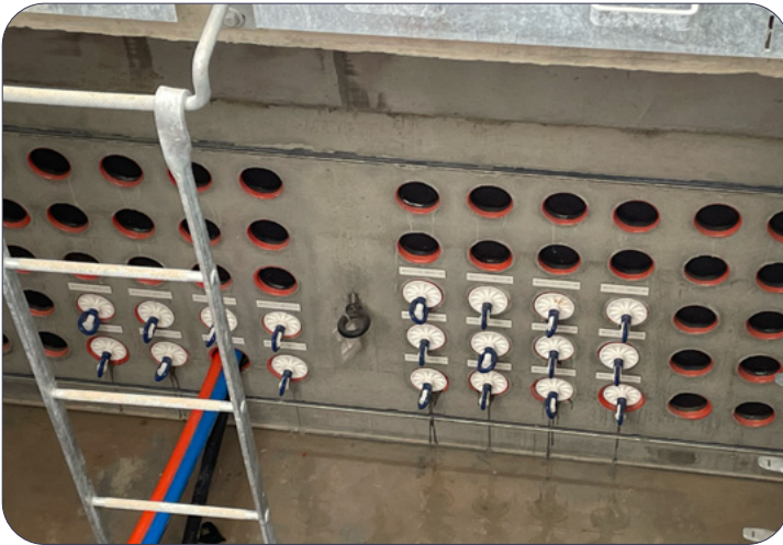
Expansion plugs installed in a vault
