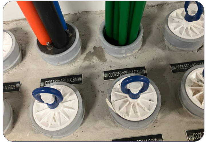
Close up of expansion plugs installed in a vault
