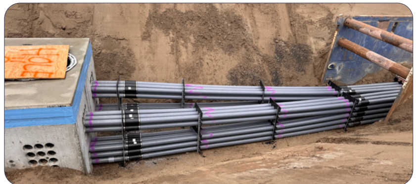
Right-to-left: transition from HDPE sticks to short PVC lengths with NS Shur-Lock Couplers before entry into vault
