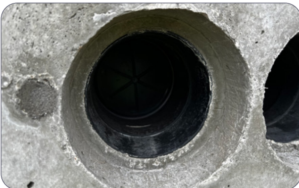
Duct entry point into a vault with insert
